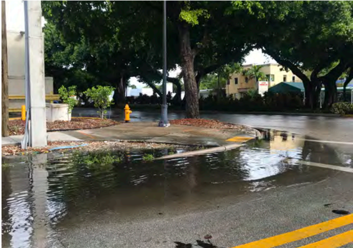
Flooded Swale at SW 16th Avenue & SW 22nd Street
