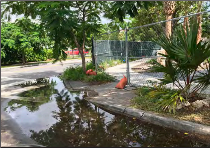
Flooded Swale at SW 21st Avenue & SW 13th Street
