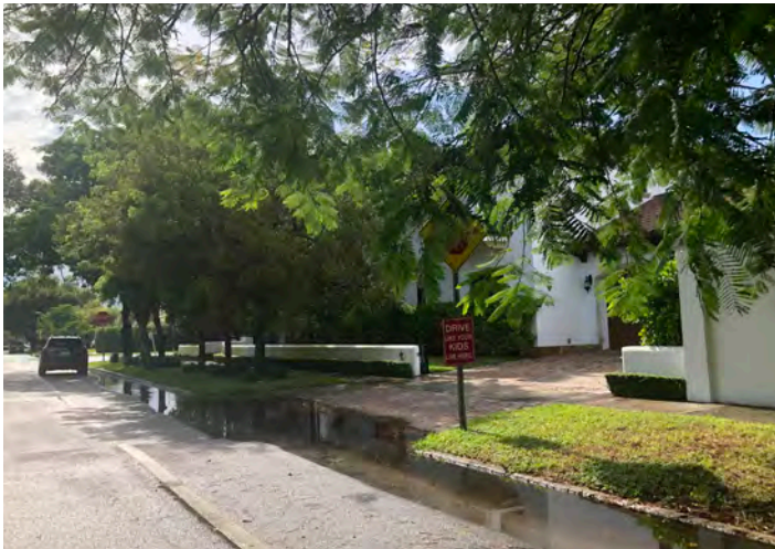
Flooded driveway and on-street parking at SW 4th Avenue.
