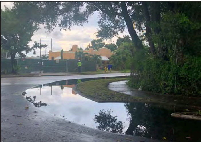
Flooded Swales at SW 10th Street Road & SW 9th Street
