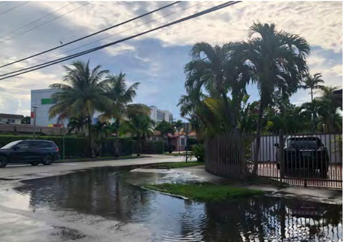
Flooded Swale at SW 24th Avenue & SW 26th Lane
