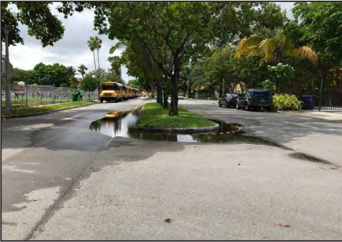
Flooded median at SW 20th Avenue & SW 10th Street
