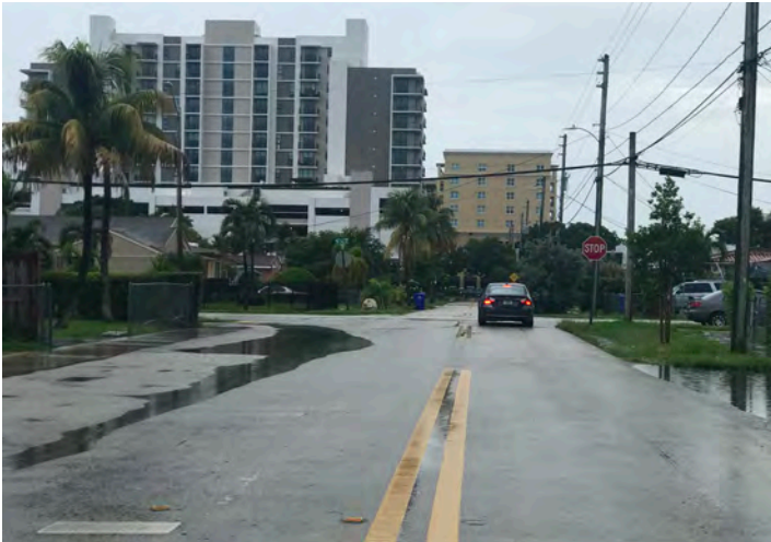
Flooded Swale at SW 15th Street
