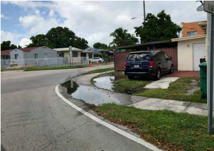
Flooded Sidewalk at SW 32nd Avenue & SW 5th Street
