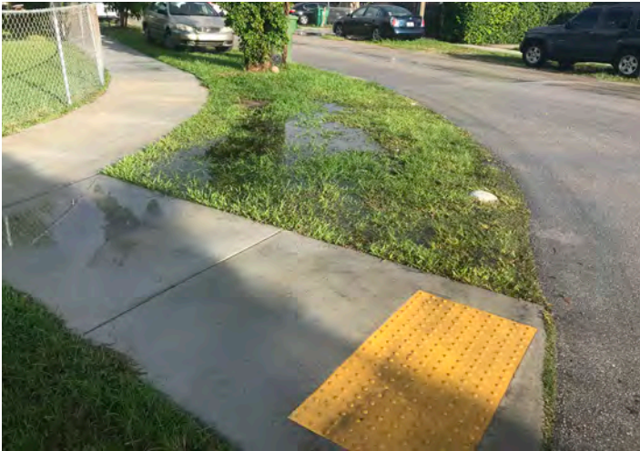
Flooded Swale at SW 26th Street & SW 34th Ave
