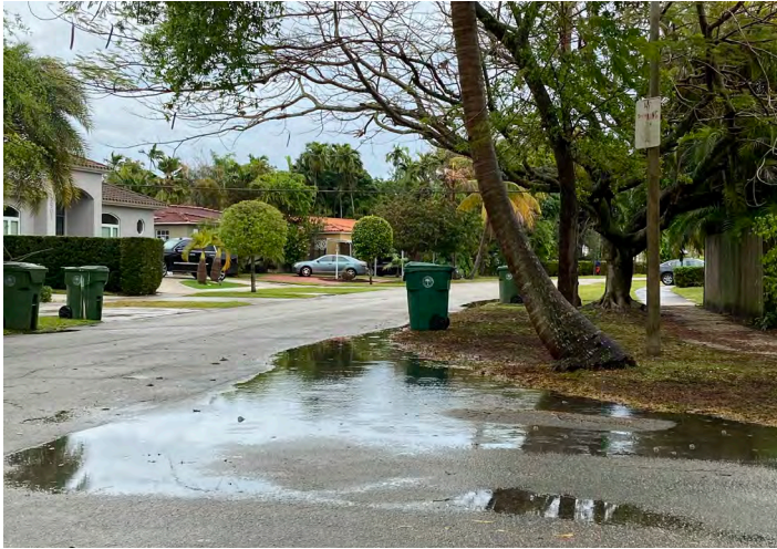
Flooded corner at SW 18 Terrace and SW 36th Avenue
