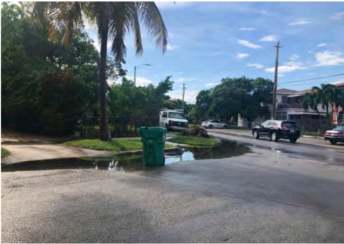
Flooded driveway and Backed up storm drain at SW 20th Road
