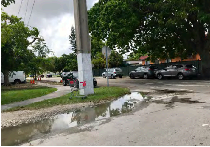
Flooded Swales at SW 29th Avenue and SW 7th Street
