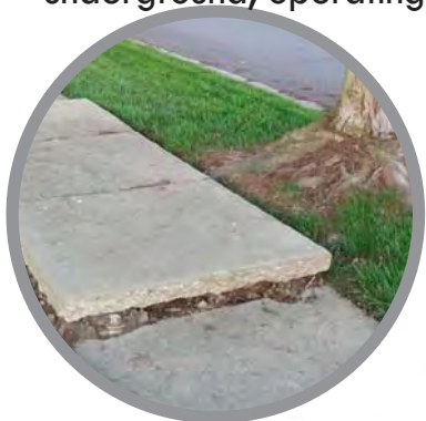
Roots uplifting pavement
