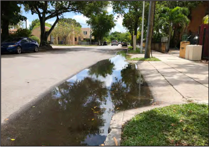
Flooded Swales at SW 19th Avenue & SW 9th Street
