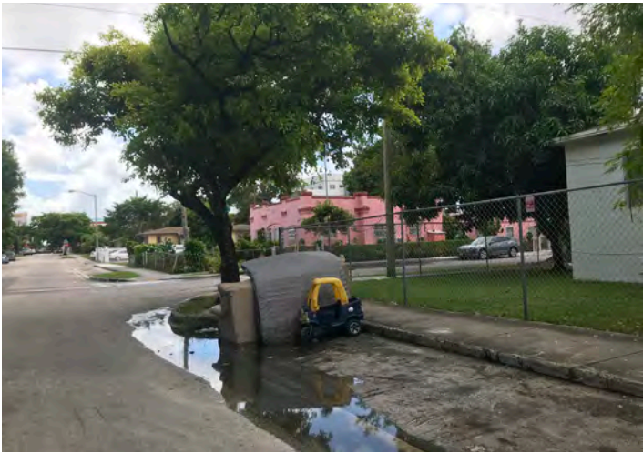
Flooded valley gutter at NW corner of SW 5th and SW 6th Avenue
