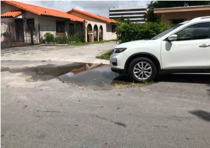
Flooded Swale at SW 29th Avenue
