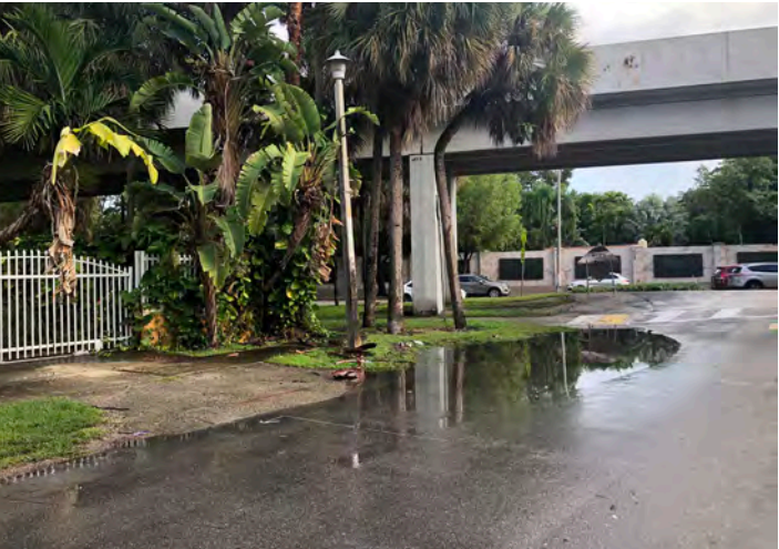
Flooded Swale at SW 19th Avenue & SW 25th Terrace
