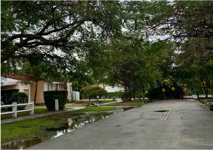
Flooded swale along Coral Gate Drive
