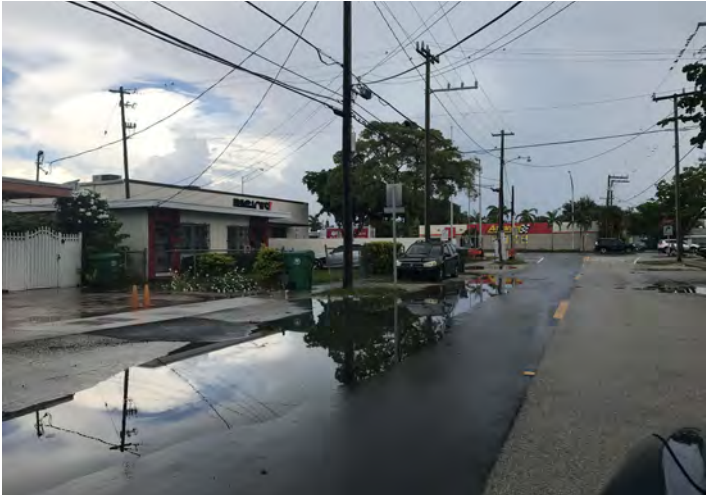
Completely paved swale with standing water on SW 21st Terrace near SW 27th Avenue
