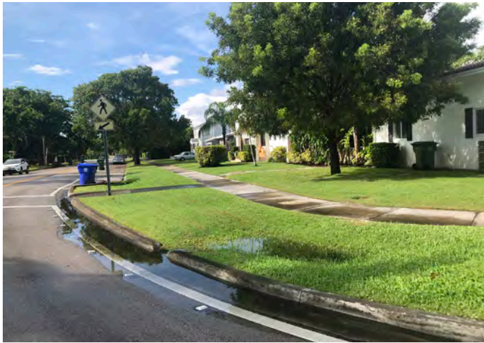
Flooding at curb cut-out gathering at low point of swale at SW 4th Avenue.
