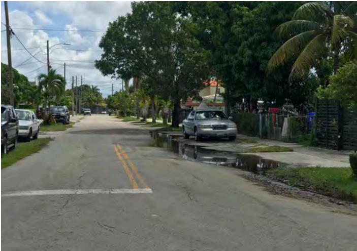
Flooded Swale at SW 30th Avenue & SW 2nd Street
