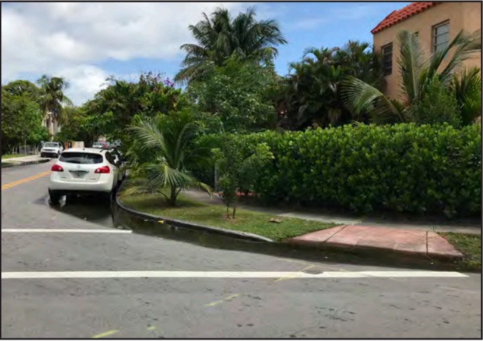
Flooded Swale at SW 19th Avenue & SW 9th Street
