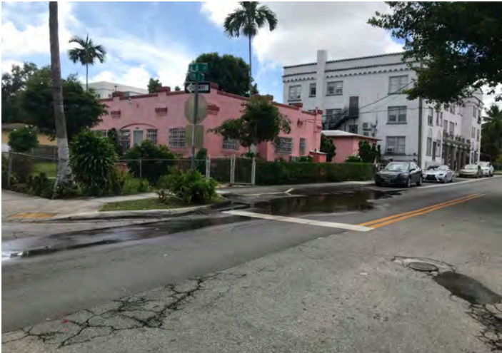
Flooded valley gutter at SW corner of SW 5th St. and SW 6th Ave.
